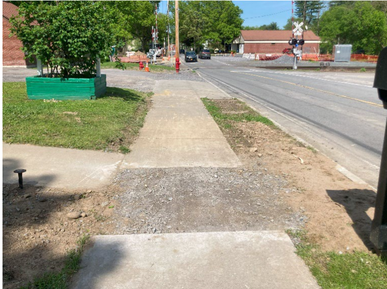
Figure 22 Sidewalk Conditions on Voorheesville Avenue Between South Main Street and Railroad Crossing, Looking North
