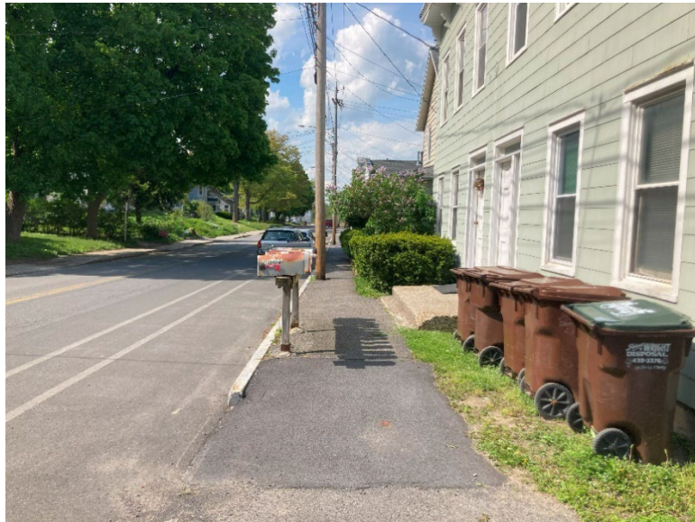
Figure 23 Asphalt Sidewalk and Accessibility Barriers on South Main Street, Looking North
